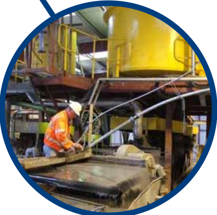
Hazardous Chemical Pumping e.g. metering cyanide solution in gold extraction
